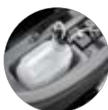
Chemical mixing system
